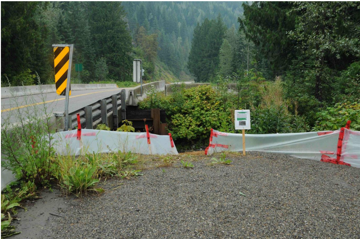
Figure 9. Temporary plastic deflection fence built in August 2015 to direct migrating toadlets on to artificial wooden bridge crossing under the Highway 31A Goat Creek Bridge.
